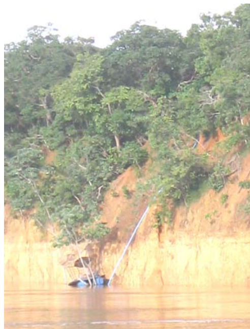
□ Image 14. Pump station for irrigation along the São Francisco River, between Pirapora and Barra do Guaicui.
